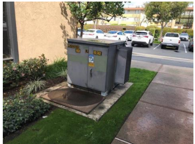
6. View of the subject property pad-mounted transformer
