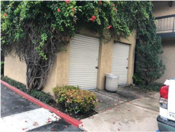
19. View of the telecommunications closet
