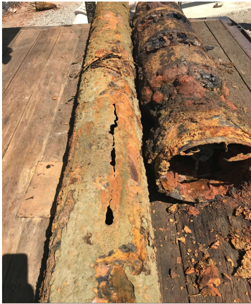
Main Plant Well 4
