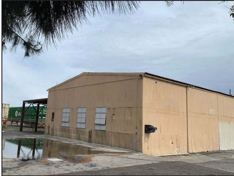
Image 7. The west and south façades of the warehouse, view toward the northeast.
