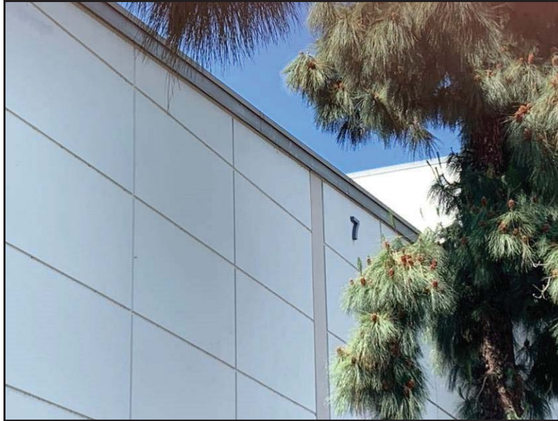
Image 17. Detail of the north façade of the addition to the west of the original building, view toward the southwest.
