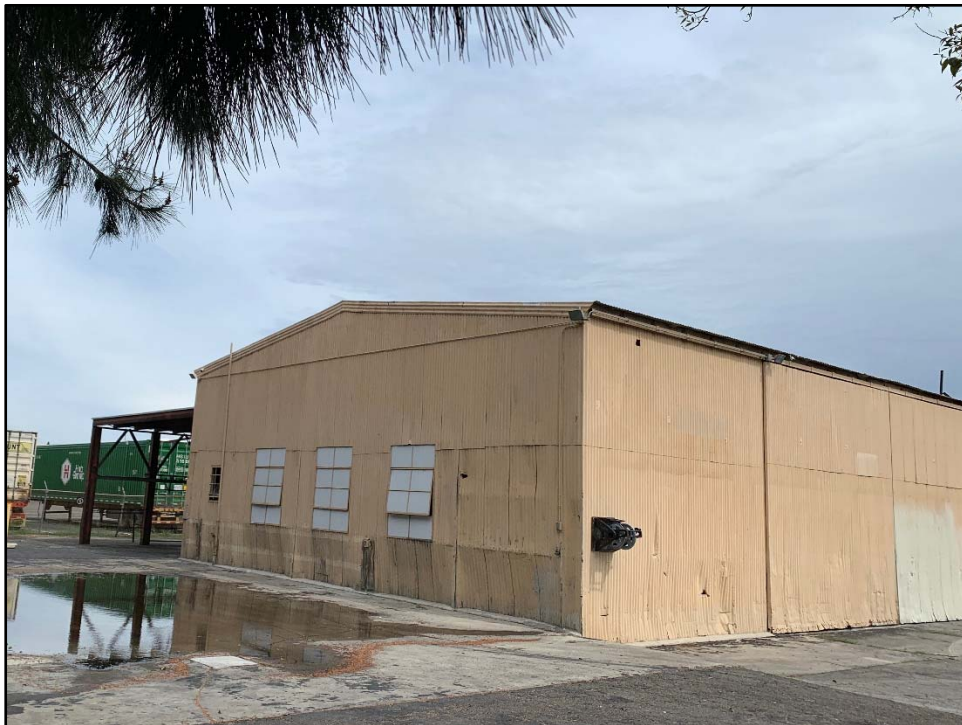
Figure 46. The west and south façades of the warehouse, view toward the northeast.
