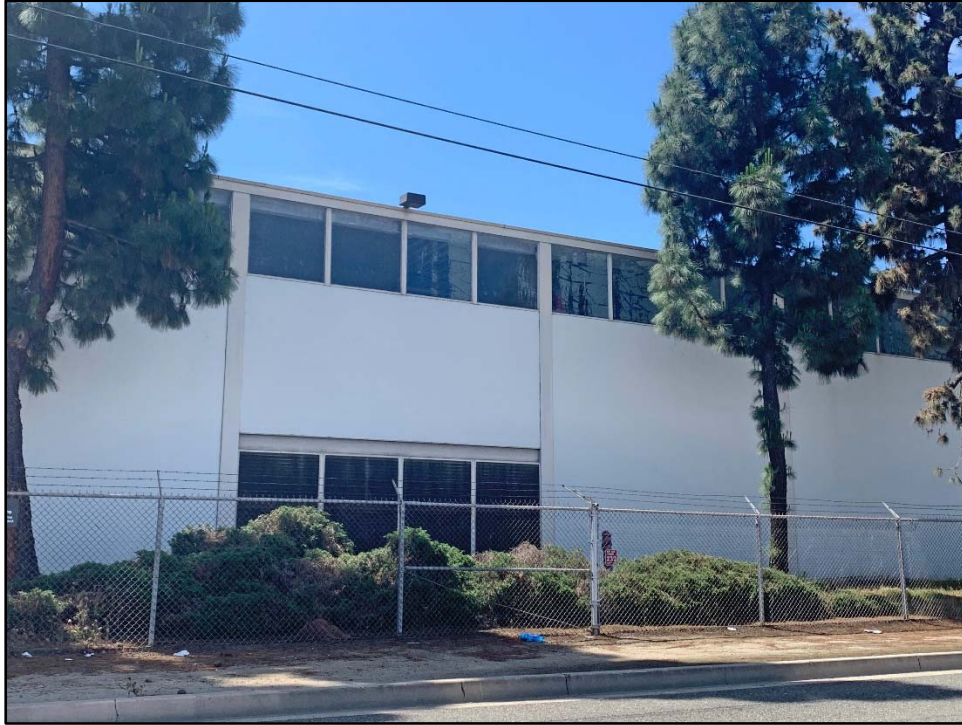
Figure 28. Detail of architectural features of the north façade of the original building, view toward the south.
