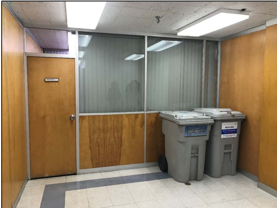
Figure 36. A typical partition off the east-west corridor of the administration section of the building, view toward the north.
