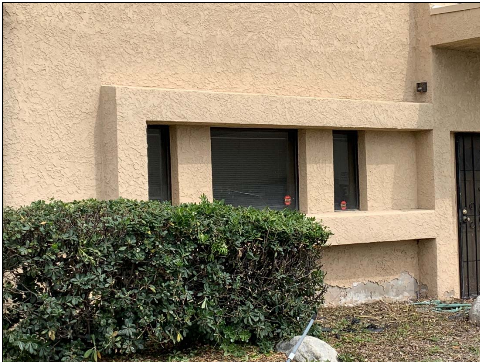
Figure 44. Detail of the windows at the south façade of the office building.
