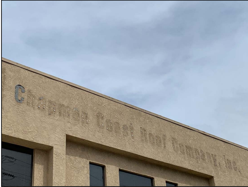
Figure 41. Detail of outline of sign at the second level of the south façade of the office building, view toward the north.
